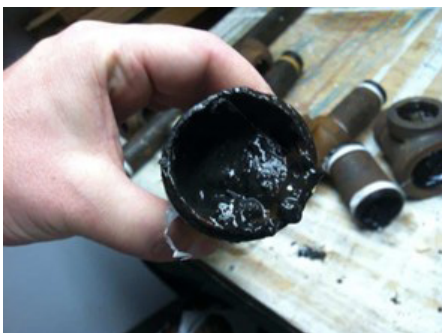
Fig 1: Heavily fouled with solids
